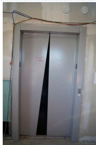
Door Jamb After FB5-DEN100 (non-functional)
